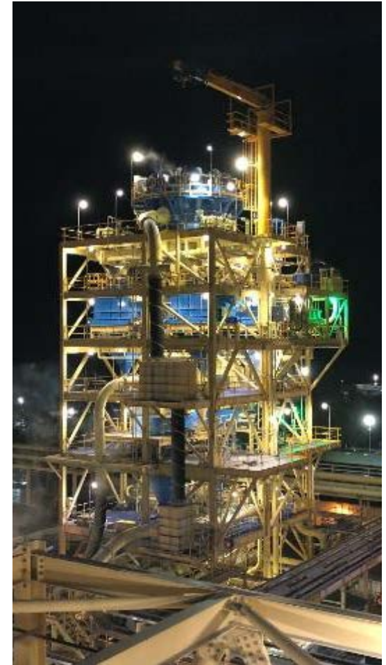
Coarse ore flotation plant, Cadia
