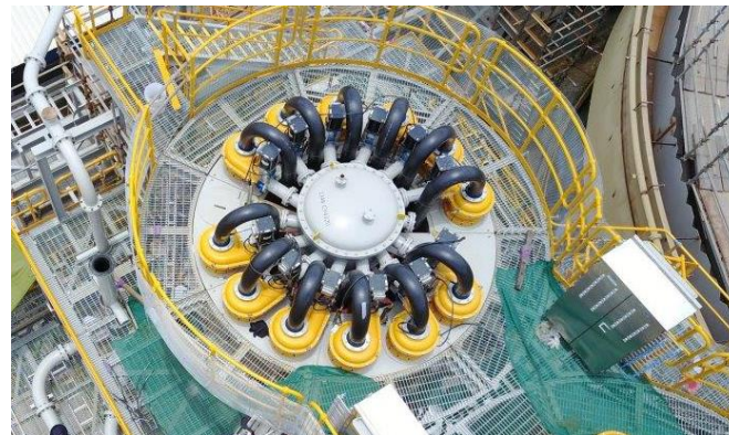
Float Tails Leach (Stage 2) cyclone and associated infrastructure
