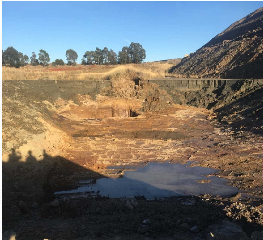
Photo B2-8: Exposed foundation on 18 th January 2018 (2018-010)
