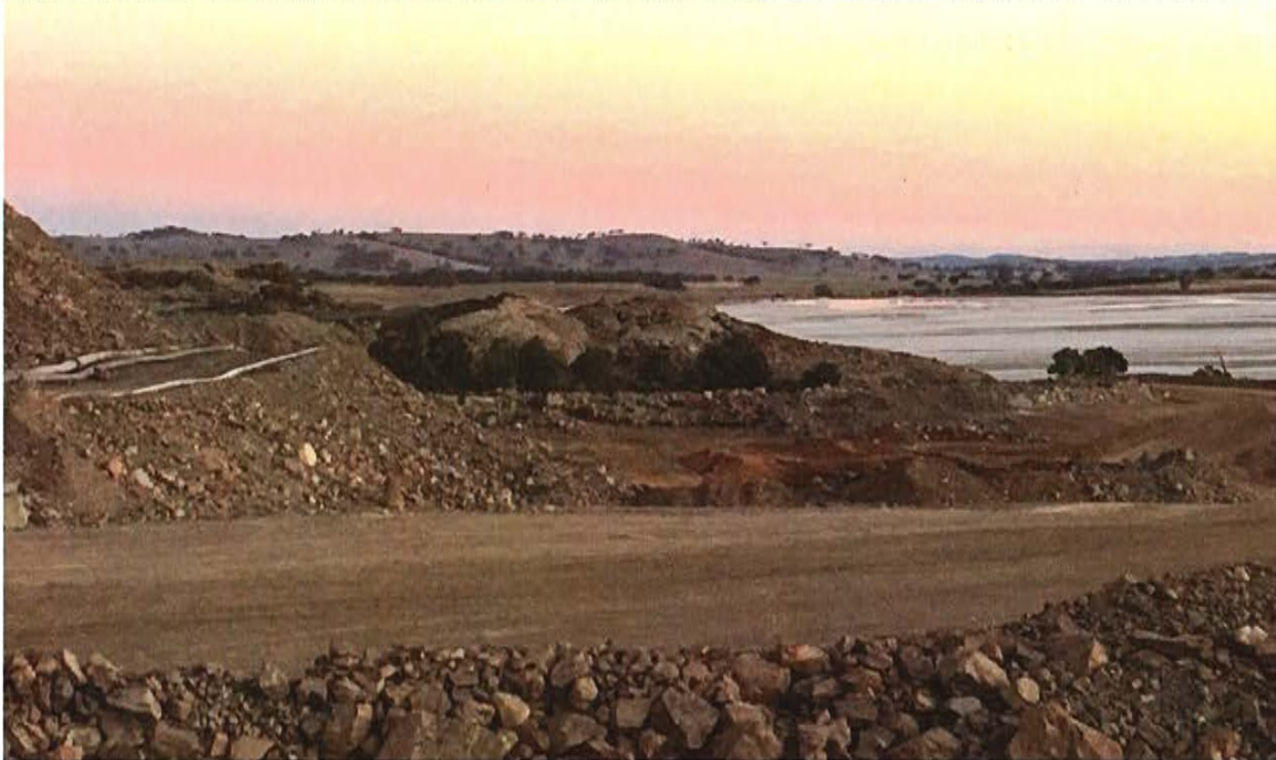
Photo looking easterly at side of slumped area (picture correction applied for low light)
