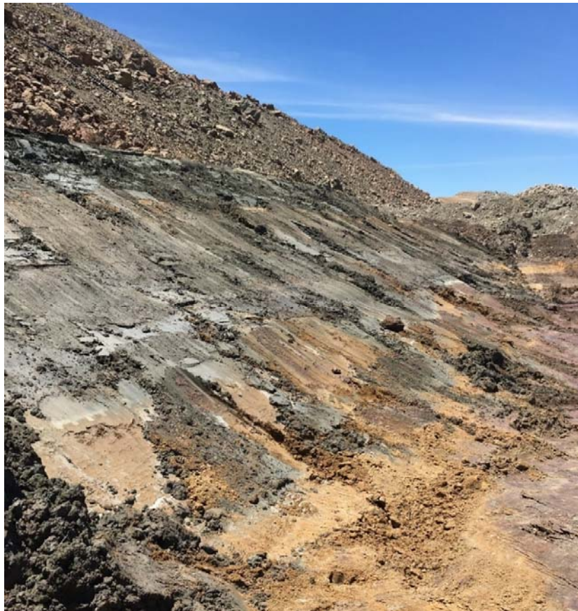
Photo B2-9: Excavated face at toe of NTSF on 17 th January 2018 (2018-011)
