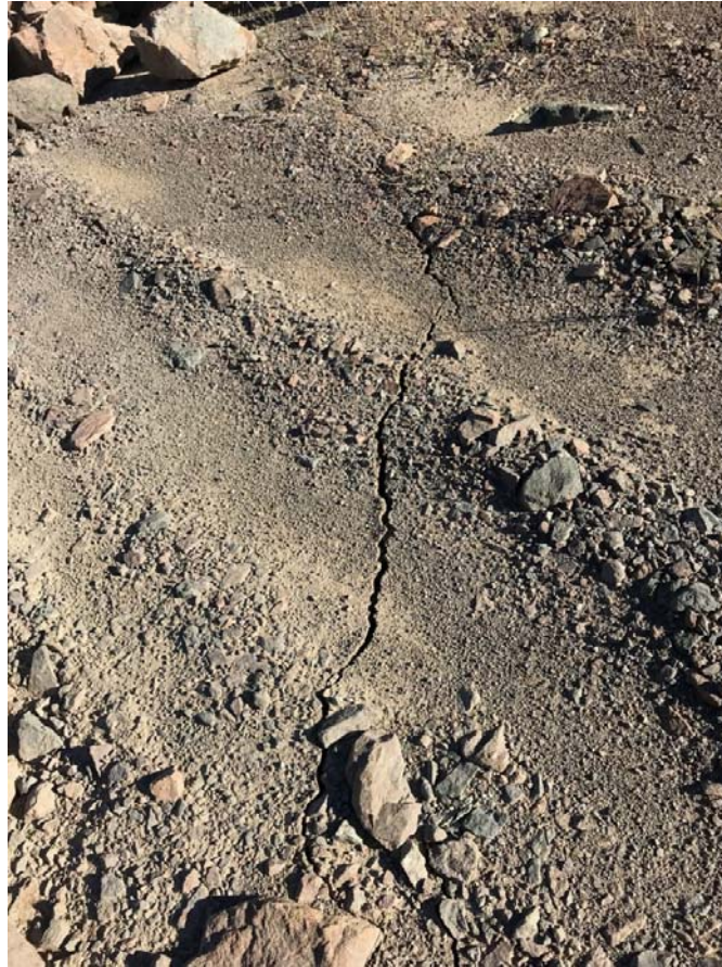
Photo B8-1: Photograph of cracking on Stage 5 crest taken at 07:48 (2018-012)
