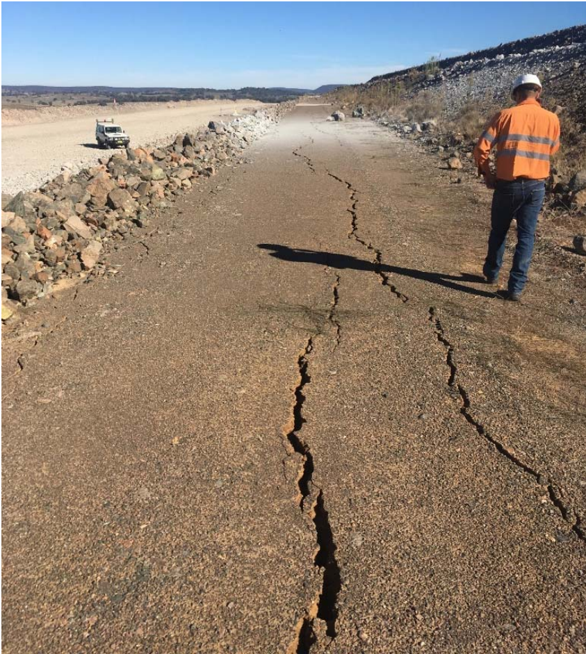
Photo B8-2: Stage 8 crest cracking looking west (2018-013)
