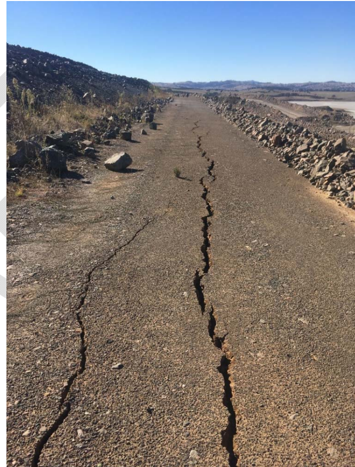
Photo B8-3: Stage 8 crest cracking looking east. (2018-014)
