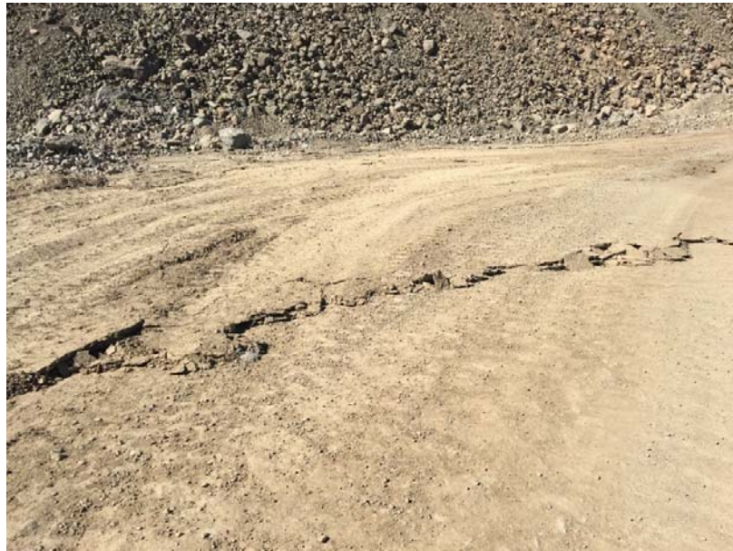
Photo B8-4: Cracking and heaving of haul road at Chainage 2060 (2018-015)
