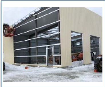
ERT Building under construction to house emergency vehicles, ERT and Iridia medical facilities
