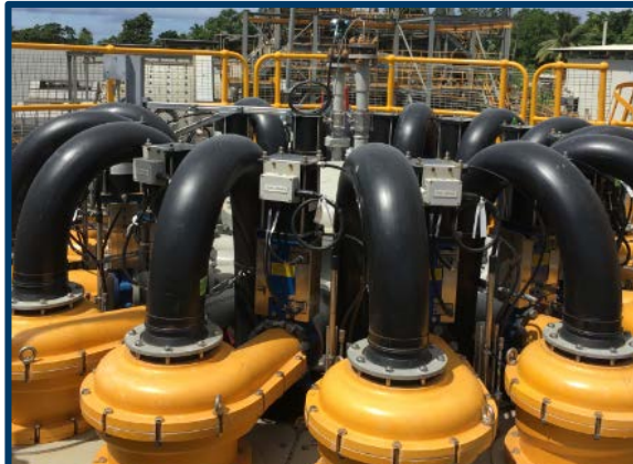
Float residue scavenging
